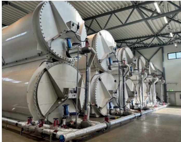
Antec was built on a new AD system that mimics the cow's digestion system
